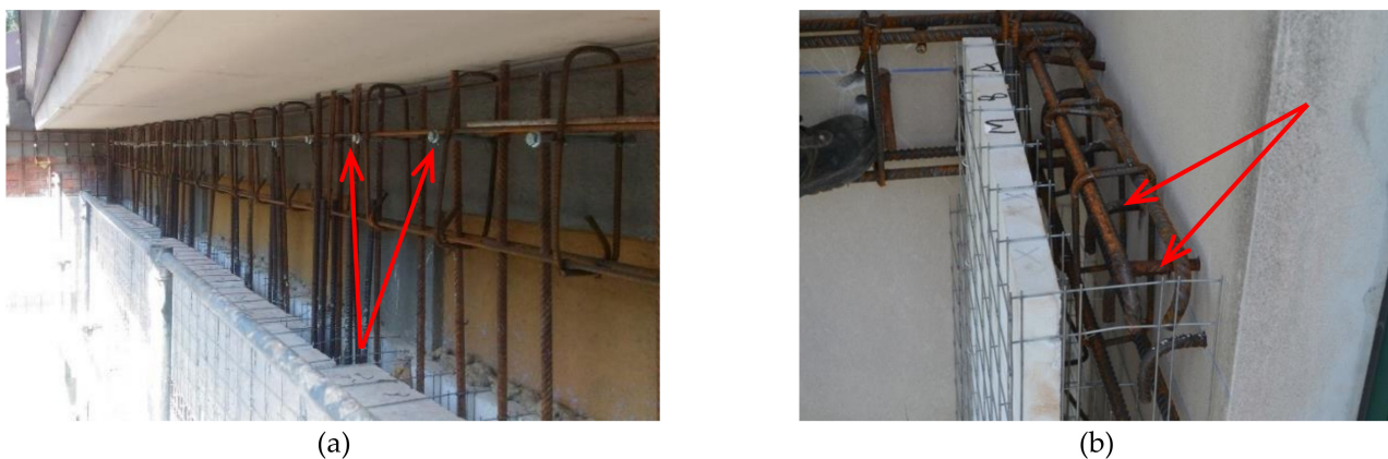
Figure 4. Connectors installed on concrete curb: (a) self-tapping concrete screws and (b) steel bars with chemical anchors.
