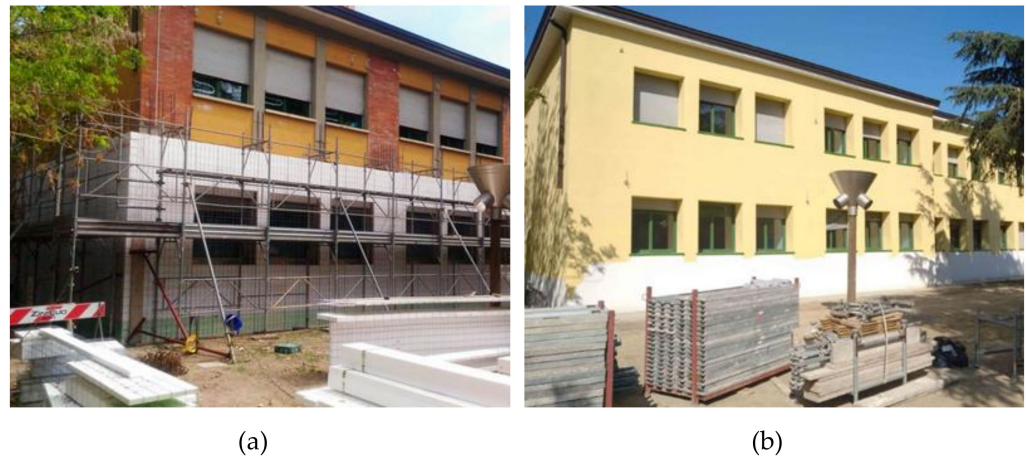
Figure 6. Installation of ICF technology on a school in Italy: (a) work in progress (b) with external finishing.
