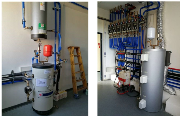
Fig. 3. Cooling tank and connection with chiller circuit (left); heating tank and secondary circuits (right).
