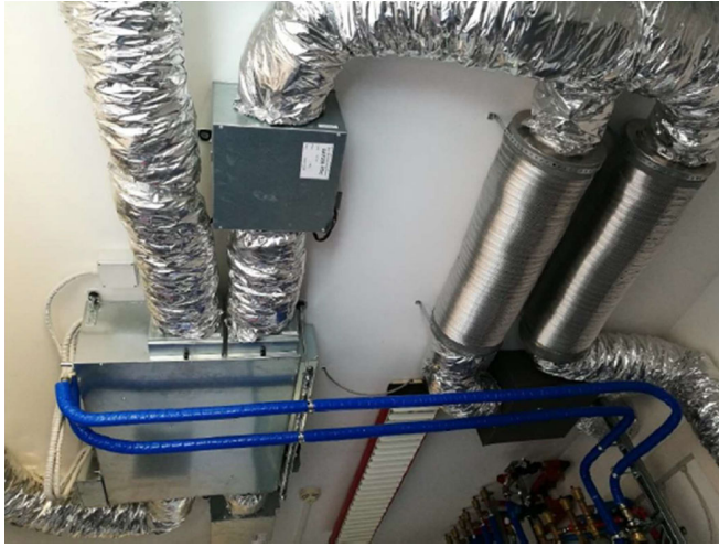
Fig. 4. Picture of the ventilation unit and connections with heating and cooling circuits (blue pipes).
