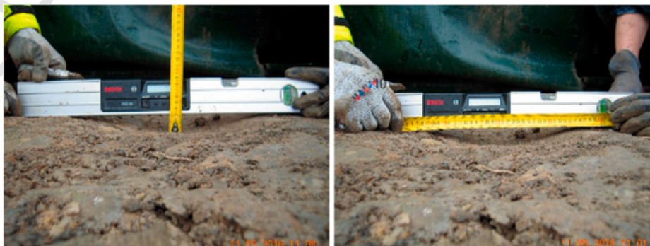
Fig. 7. Macro irregularities and depressions on the slope surface.
