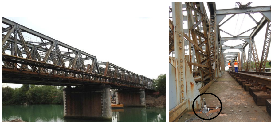
Figure 4.58 View of Musile bridge and sensor installation on it.
