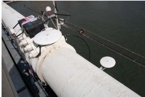
Figure 4.104 A typical GPS antenna and accelerometer installation.
