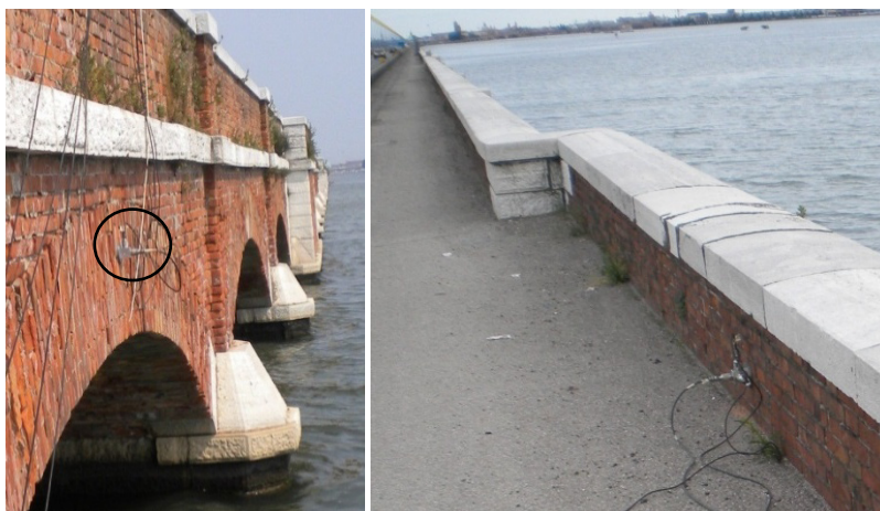
Figure 4.44 Sensor installation on the structure.
