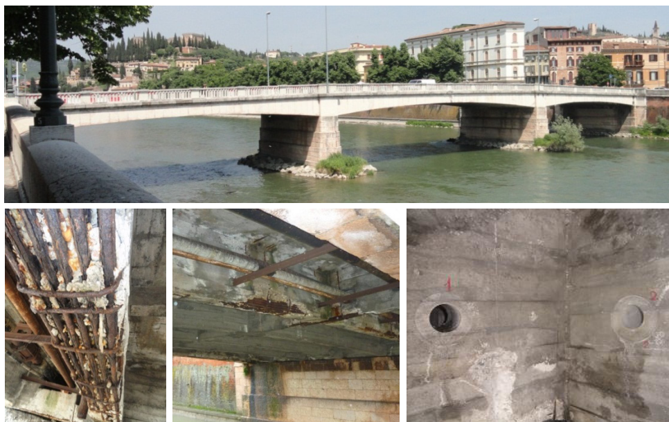
Figure 4.81 View of the People's New Bridge and the damaged elements.
