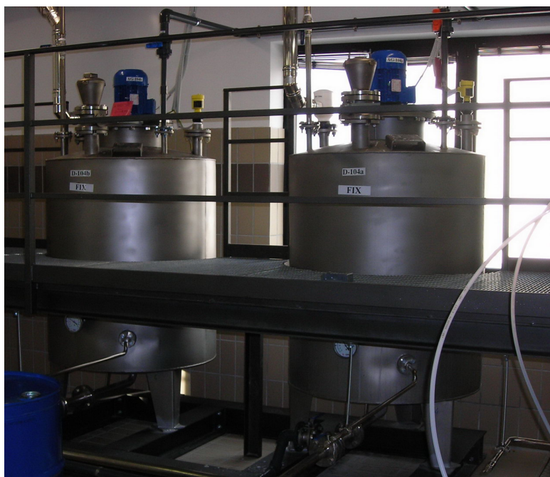
Figure 3.5: Two of the buffer tanks for chemicals at ground floor of Lab1.
