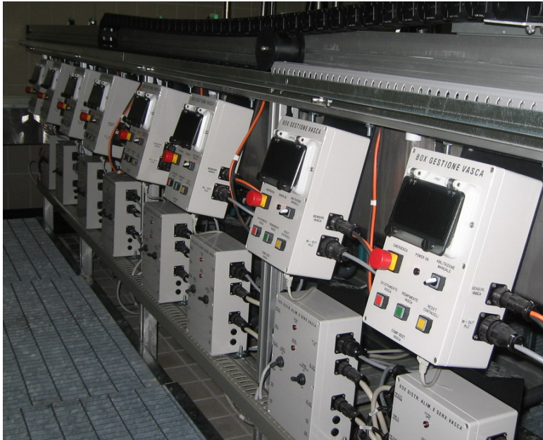
Figure 3.9: Photograph of PLCs controlling the tanks of one development line.
