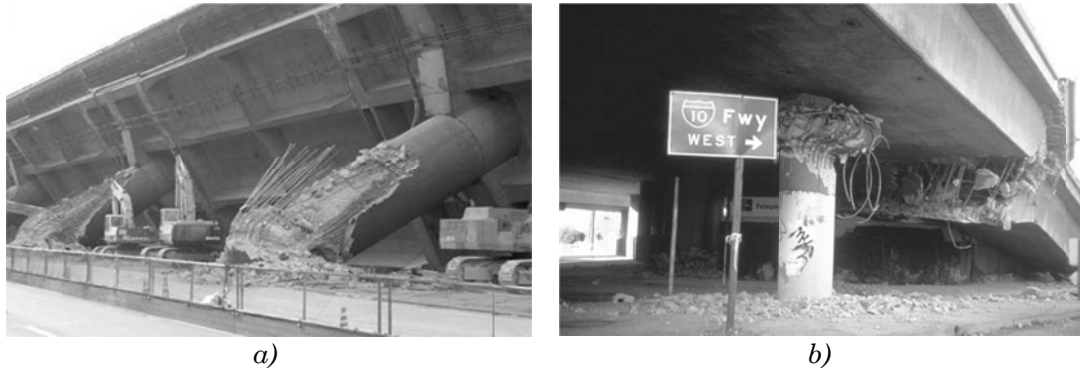
Fig. 5.1 – Shear failure in reinforced concrete piers: a) Hanshin expressway, Kobe earthquake, Japan, 1995, b) Northridge earthquake, California, 1994
