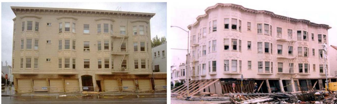
Fig. I.8 – S. Francisco soft-storey building damage – Loma Prieta earthquake 1989 [I.12]
