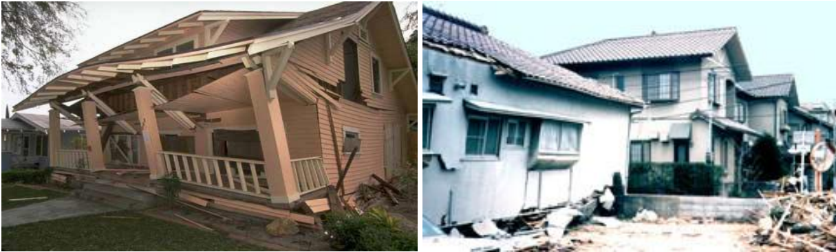
Fig. 1.1 - Destruction of a residential house after Northridge earthquake 1994 [1.5] (left) and Kobe earthquake 1995 [1.6] (right)
