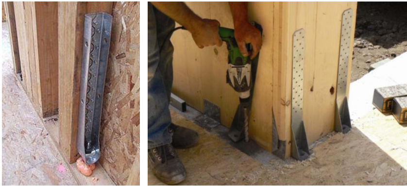
Fig. I.7 – Typical anchorage system of Platform Frame building (left) [I.11] and CLT building (right) [I.9]
