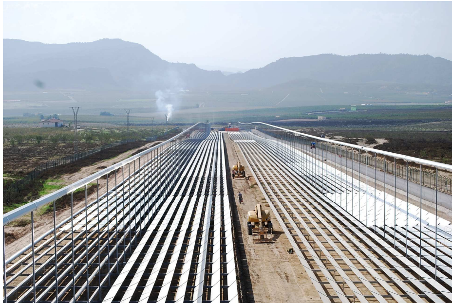
Figure 7. SPP with Fresnel technology.
