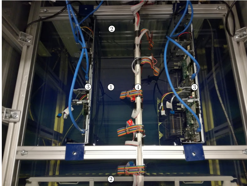
Figure 6.4: Top view of the vessel, with: the mineral oil (1), the immersed heat exchangers (2), the servers (3), and the matrix of thermocouples (4).
