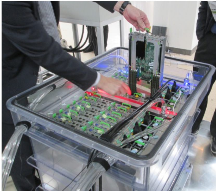
Figure 1.14: Snap shot of a liquid immersion cooling system with natural convection, Matsuoka et al. (2017) .
