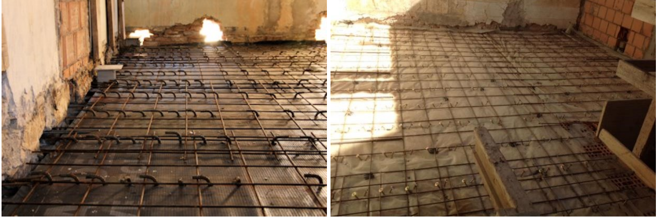
Fig. 1.2 – Renovation of existing timber floors with mechanical connectors before realization of the concrete slab.
