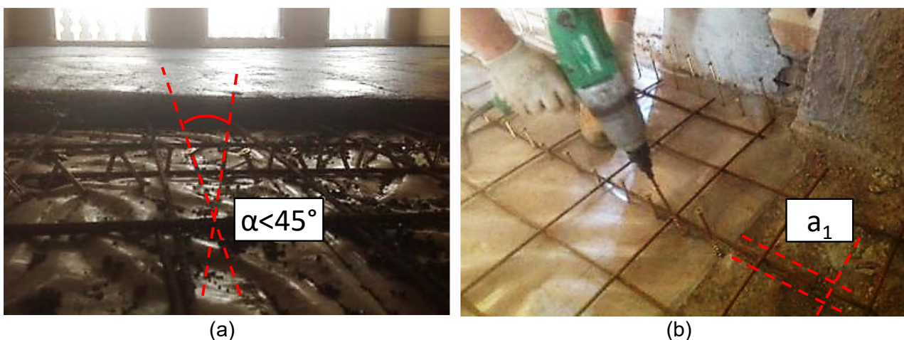
Fig. 2.1 – Issues that might occur throughout the installation of many screws with an angle respect to the grain.
