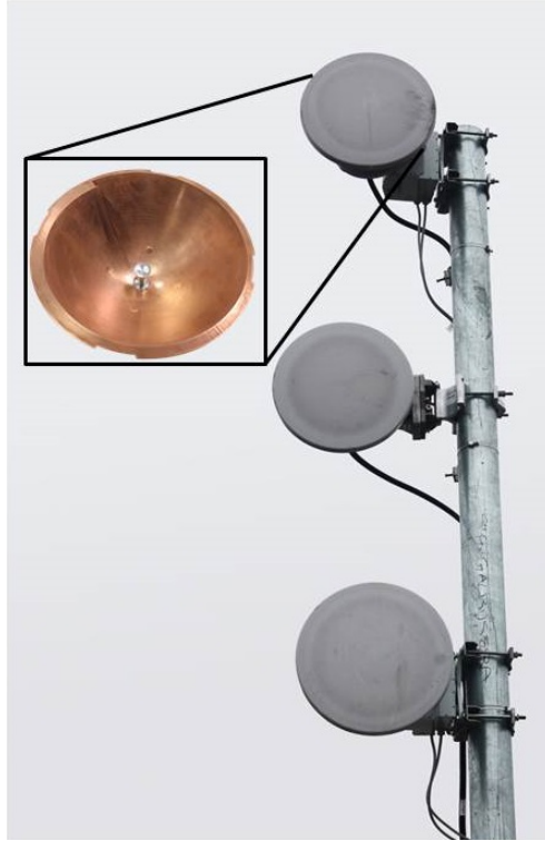
Figure 3.3: Example of transmission side of the link with three parabolic antennas installed on a pole. \ell = \pm 1 antennas are on the top and on the bottom, respectively. Inset: picture of a twisted \ell = +1 antenna without radome.
