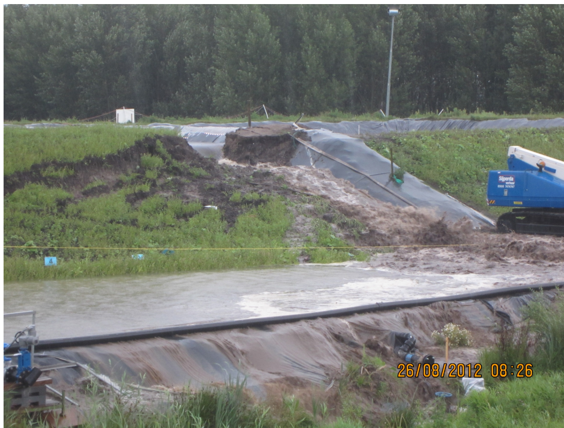
FIGURE A.29: Breaching of the dike
