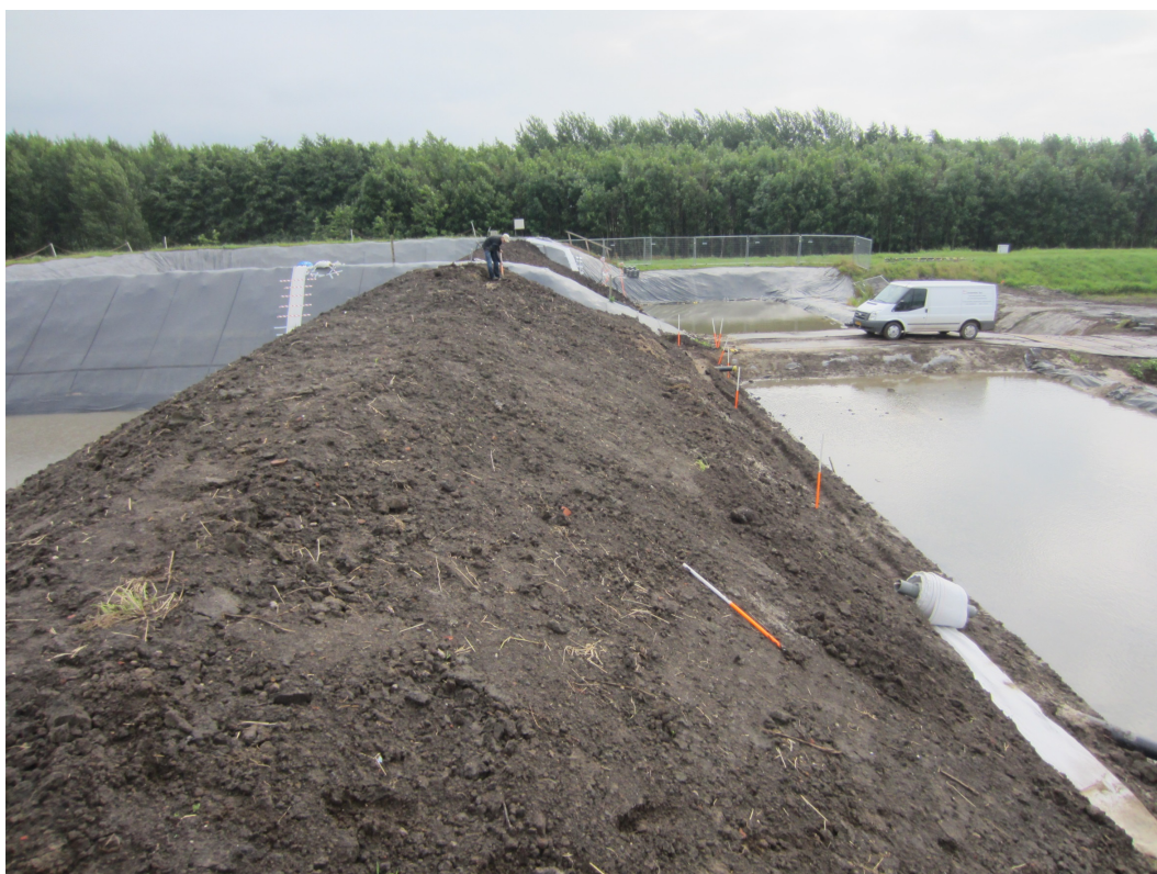
FIGURE A.16: Installation of the optical fibres in a trench on the downstream slope
