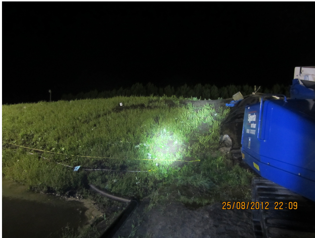
FIGURE A.25: First sliding of the downstream slope
