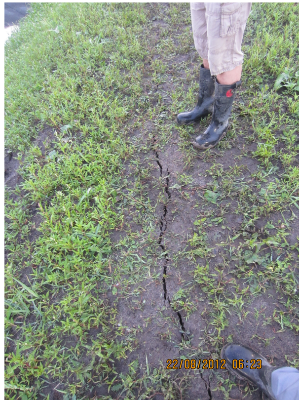
FIGURE A.23: First crack appeared on the crest
