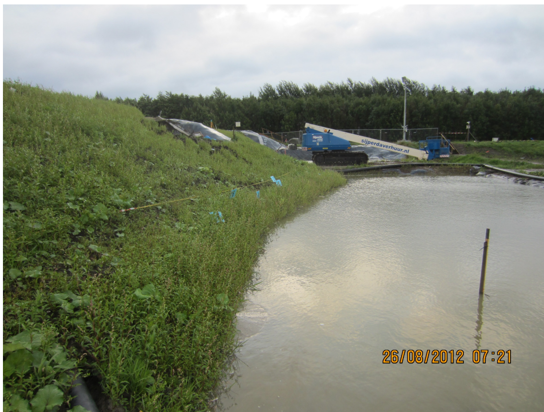
FIGURE A.28: Further buldge of the downstream toe
