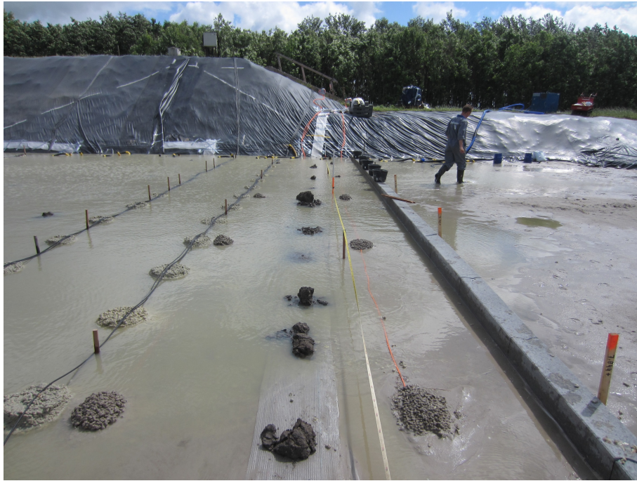
FIGURE A.9: Installation of pore pressure sensors and optical fibres at the dike base.
