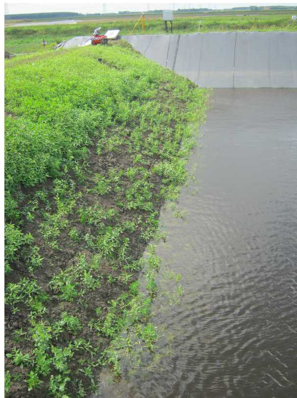
FIGURE A.24: Cracks on the upstream slope
