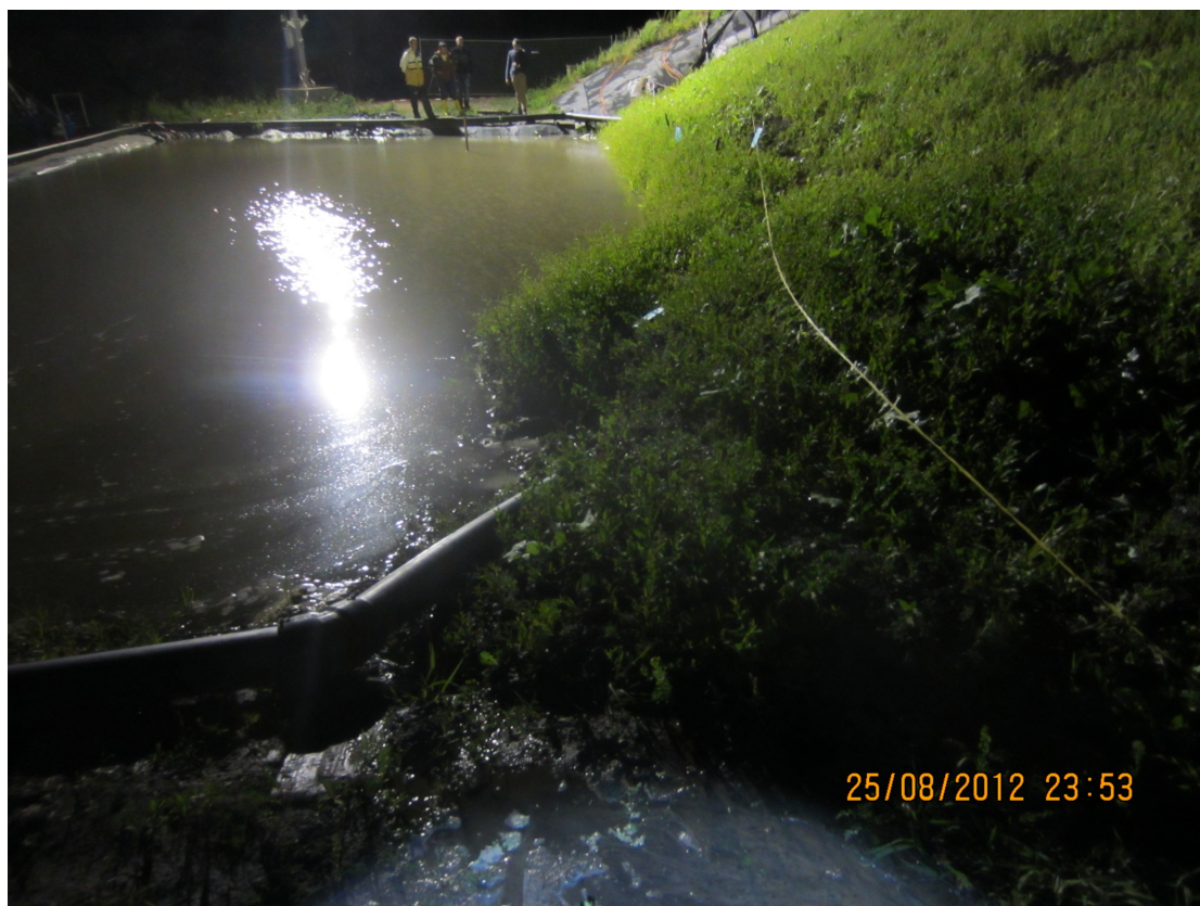
FIGURE A.26: Buldge of the downstream toe
