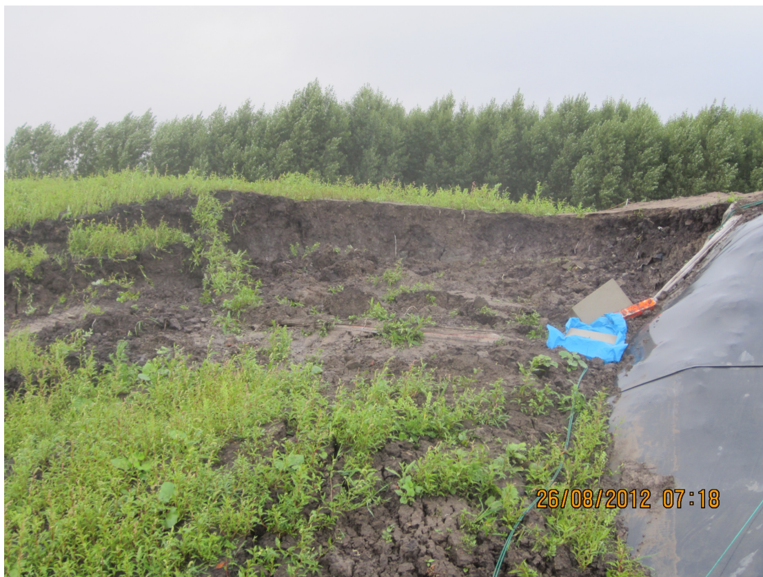
FIGURE A.27: Further sliding of the downstream slope
