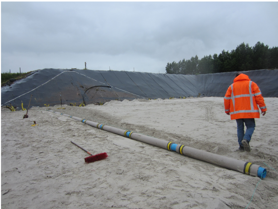
FIGURE A.8: Installation of the controllable drainage tube, surrounded by a sand filter.
