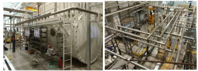
Figure 11. View of the on-going assembly of MITICA cryogenic plant—auxiliary cold box (left) and piping layout inside the building for auxiliaries (right).
