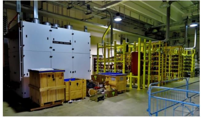
Figure 1. SPIDER accelerator power supplies: left, dummy load; right, insulating frames with pulse step modulator modules.
