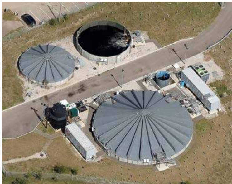
PLATE 3: Masons Leachate Treatment Plant, Ipswich, UK.
