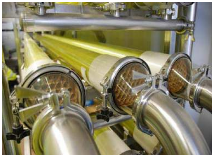
PLATE 4: UF Membrane Tubules at Masons Leachate Treatment Plant.
