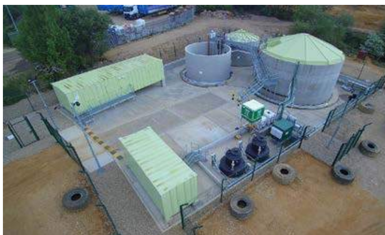
PLATE 1: View of Hatfield Leachate Treatment Plant, showing fully bunded area, chemical dosing compound in right foreground, and control building at the rear left.
