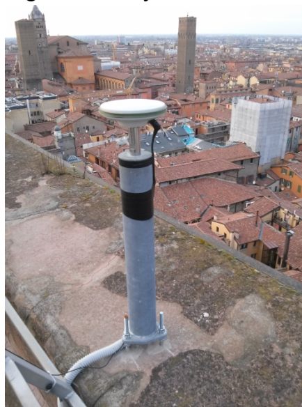
Figure 3 – The BOGA GNSS antenna installed on the top of Garisenda tower by the DICAM department since 2013.
