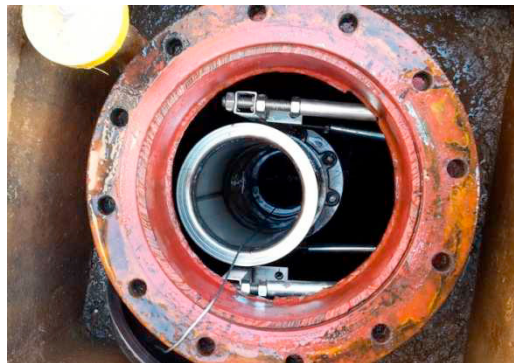
Figure 3. Insertion of a 12 m length tube inside the injection well to favour the injection of water and thus avoiding bubbling and excessive oxygenation
