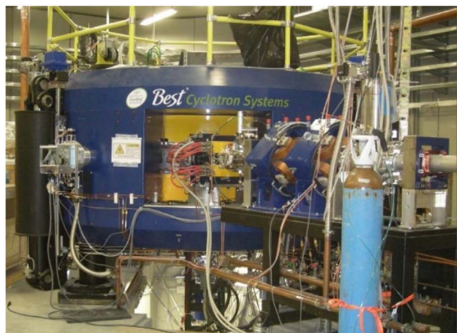
Fig. 1. BestC70 cyclotron recently installed at LNL in the SPES building.
