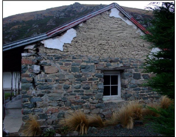
Figure 4: Hakatere Station (1862) greywacke rubble walls with mudstone gables. Lack of bond between walls with activation of out-of-plane mechanism.
