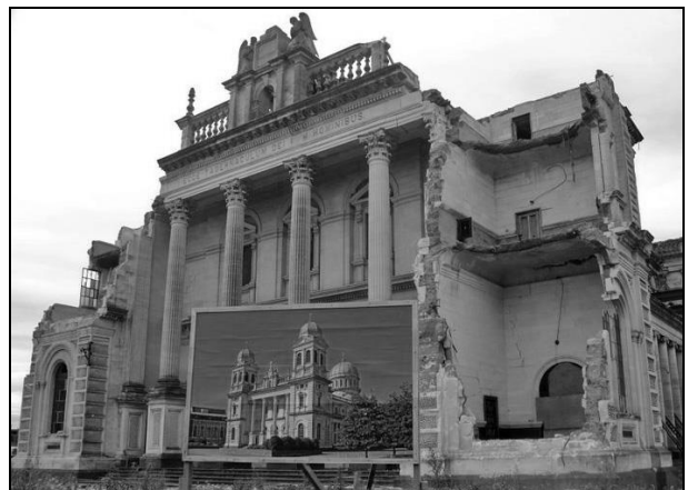
Figure 6: Cathedral of the Blessed Sacrament (1899), Christchurch. Oamaru limestone facing with cast in-situ no-fines concrete core walls. Collapse of the towers due to inadequate lateral resistance of the masonry walls.
