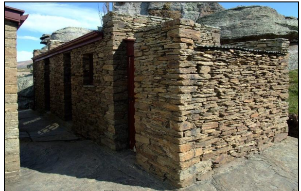
Figure 23: Mitchell's Cottage - outbuilding, Fruitlands, built in 1904 by the owner using local schist.
