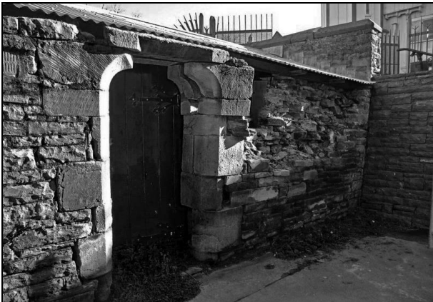
Figure 2: Canterbury Provincial Council Buildings, Bellamy's (1864). 3 leaf basalt (from Banks Peninsula) wall and limestone ornamentation. In-plane failure shown by diagonal cracking (highlighted for clarity) and twisting of the buttress.
