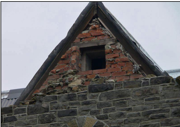
Figure 3: Canterbury Provincial Council Buildings, Bellamy's (1864). Halswell basalt facing with clay brick backing wall. Out-of-plane partial collapse of a gable due to the absence of bond between leaves.
