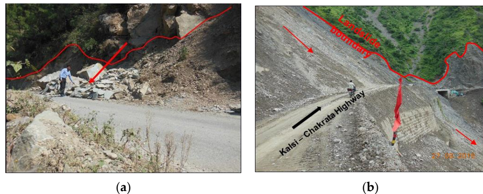
Figure 2. Active landslides along the Kalsi-Chakrata road corridor, (a) Rock Fall between Chapanu and Sahiya, (b) Amroha landslide site in 2017, retaining wall damaged.
