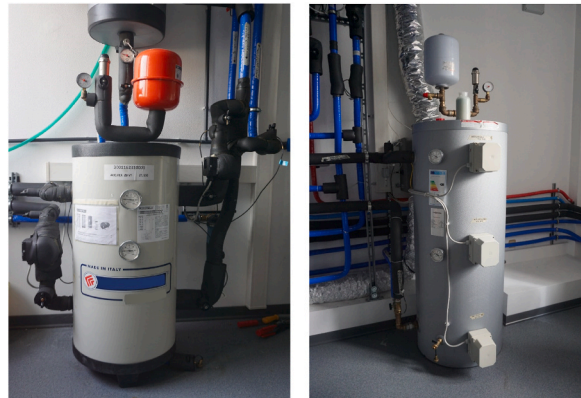
Fig. 4. Cooling (left) and heating (right) tanks.
