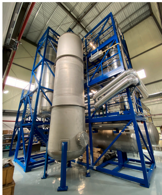
Fig. 2. Distillation plant installed in the Overground LS building at the JUNO site.
