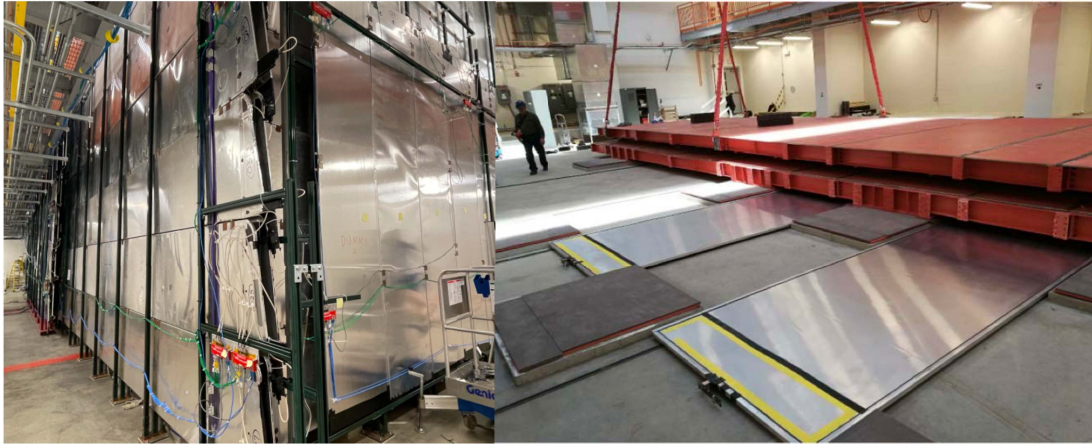
Figure 3.17: Left: Picture of the Side CRT south and west walls seen from the ICARUS building ground pit. Right: Fully installed Bottom CRT module during the warm vessel deployment. Photos from Ref. [140].
