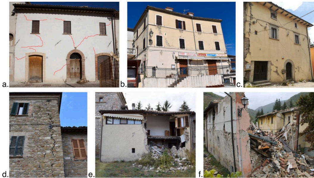
Fig. 10. Examples of EMS-98 damage grading to buildings within the dataset: a) D1; b) D2; c) D3 with severe shear cracks; d) D3 with triggering of a façade overturning; e) D4; f) D5.
