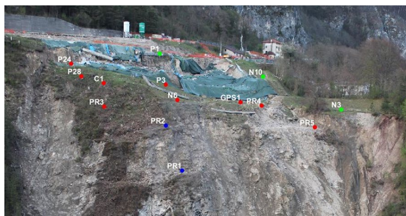
Figure 13. Image of the landslide taken on 3 May 2021 from the camera's point of view with the topographic target location. The blue dots (PR1 and PR2) correspond to the targets destroyed in the collapse of June 2021, the green ones (N3, P1, and N10) to areas where movements are very low, and the red ones highlight the targets characterized by a high movement rate.
