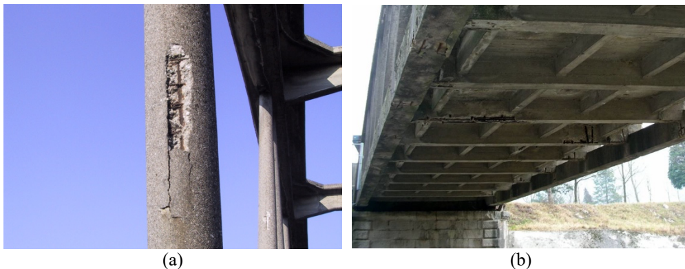
Figure 5: Spalling of concrete and corrosion of exposed rebars on: a) r.c. hanger and b) deck [25].
