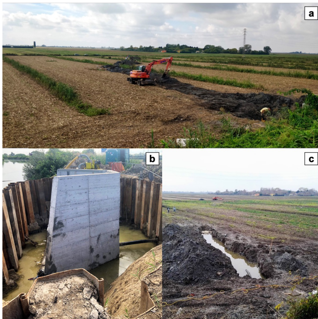
FIGURE 2 | Pictures of the experimental infrastructure: The drainpipe path along the experimental field after the trench digging and the corrugated polyethylene drainpipe establishment (a), the intake (b) and the excavation after soil piping occurred in preliminary tests carried out in 2020 (c).
