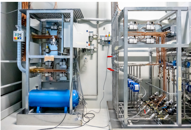
Fig. 1. The SPES Front-End hydraulic and pneumatics control circuits located in the pre-bunker (S017).
