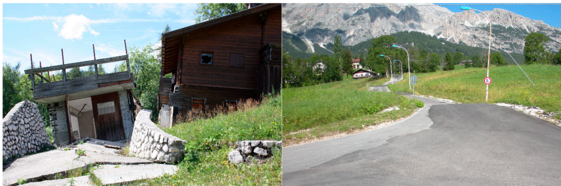
Figure 2. Buildings damaged and roads disrupted by the movement of the Rio Roncato landslide.
