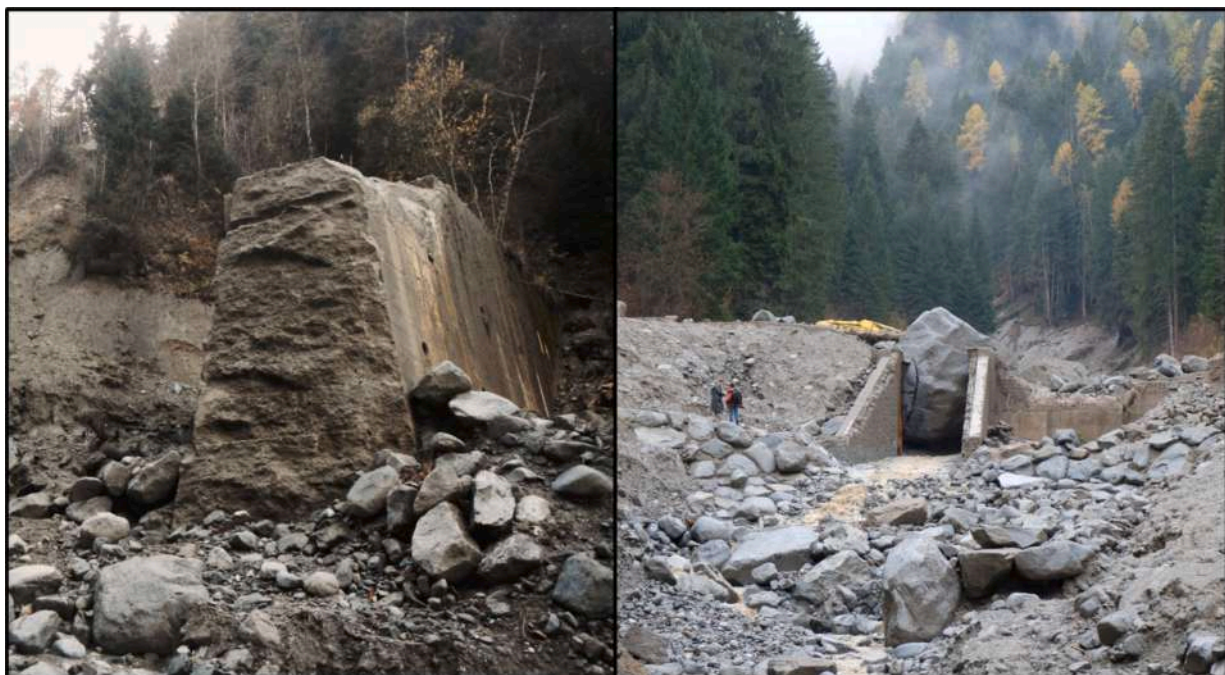
Fig. 4. Check dam failure (left panel) and obstruction of the opening of a sediment trap by a large boulder (right panel). Both the pictures were taken after the disastrous event of the Rio Rotian reported in section A.1.
