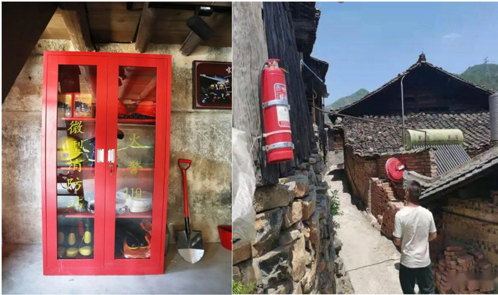
(e) Partial fire protection in the Hexinwu Building Complex
