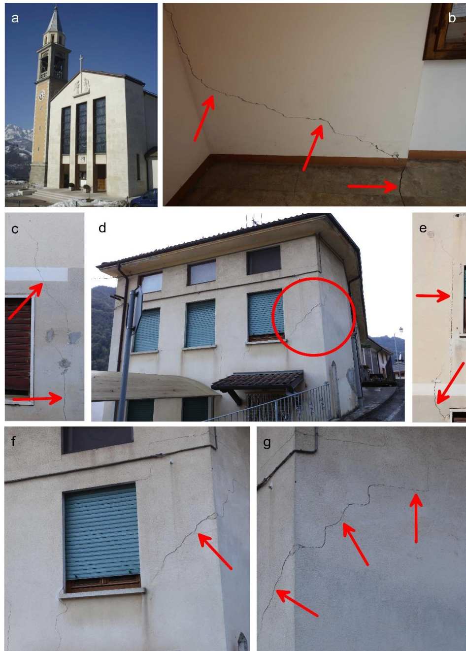
Figure 2. Pictures of Roveglia Church (a) and one of the most damaged buildings in Cappellazzi district (c–g). In (b), a large crack in the portico of the church is shown.
