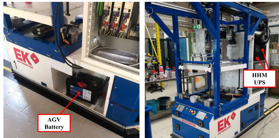
Figure 3.14: The HHM prior to the hardware upgrade: old AGV batteries (on the left), the HHM UPSs (on the right).
