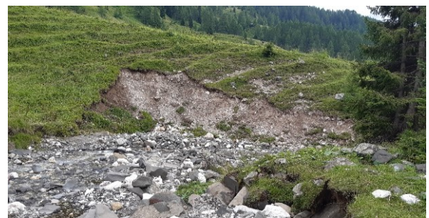
Fig. 2 – Bank erosion and channel widening featured by the Rio Cordon during the Vaia storm.
