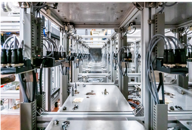
Fig. 4. Cabling of the mechanical limit switches used to detect the TIS unit presence within the storage rack.
