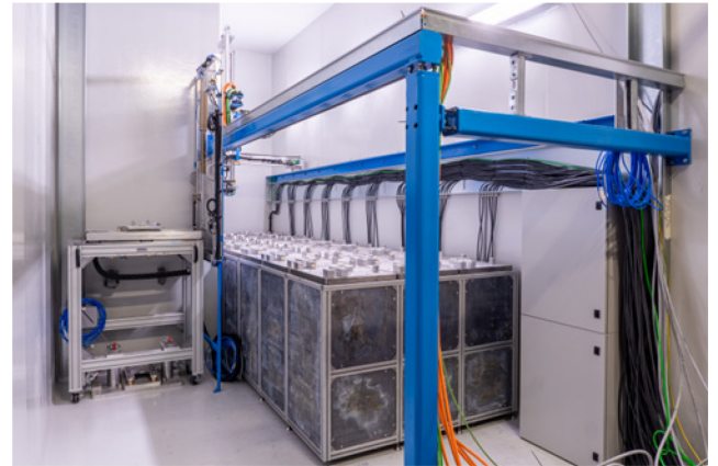
Fig. 2. The Temporary Storage System (TSS) installed in the SPES target area (S041).
