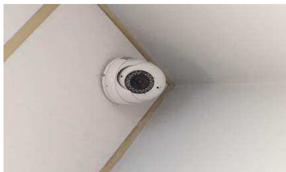
Pic. 10: '...a contrast between trying to create a welcoming environment and...trying to protect people... trying to create the health and safety systems within the building that keep people safe' . [Ireland, TS]
