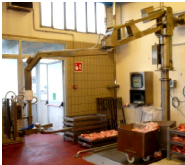
Figure 2.45 Semi-automatic manipulator in the blending area.
