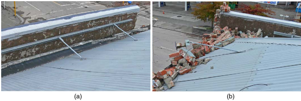
Figure 22. Performance comparison between parapets braced back to a structural element with and without a horizontal steel strip: (a) with a horizontal steel strip; (b) without a horizontal steel strip.
