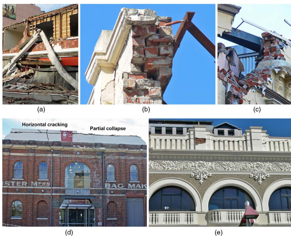
Figure 21. Typical examples of observed failure mode for adopted retrofit interventions: (a) collapsed concrete beam; (b) bracing back to structural element – short embedment of the adhesive anchors; (c) steel strip; (d) bracing back to structural element – cracking above the horizontal steel strip (highlighted in black); (e) steel strip – cracking above the horizontal steel strip.
