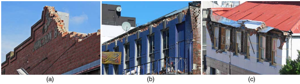
Figure 15. Examples of failure categories considered in collapsed parapets: (a) partial parapet collapse; (b) parapet collapse; (c) parapet and wall collapse (braced parapet).
