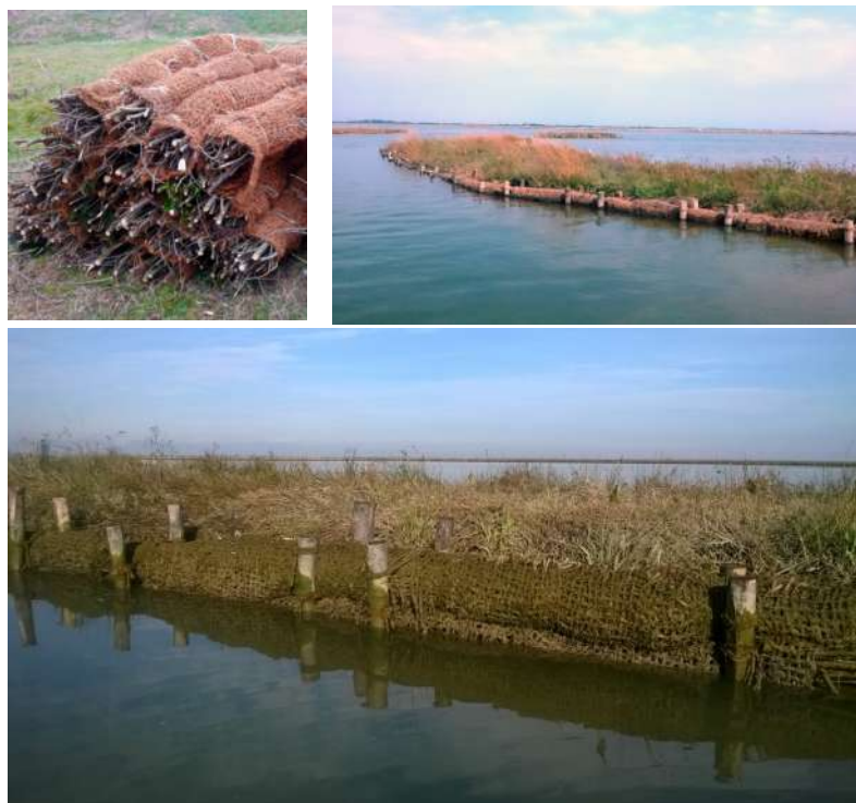
Figure 2. Examples of fascines produced locally (upper left) and then placed to protect salt marsh edges from erosion in LIFE VIMINE (upper right and bottom).
